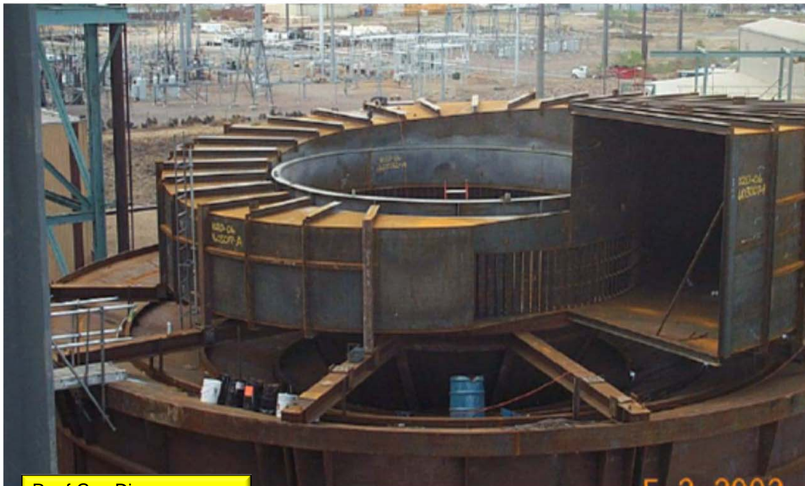
Roof Gas Disperser
